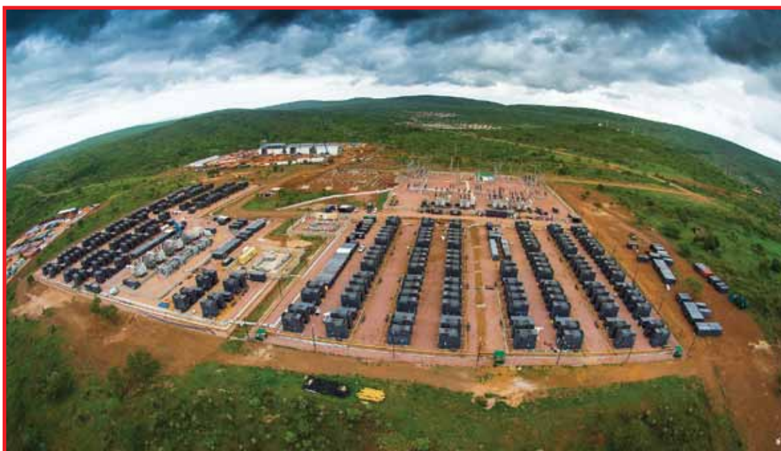
235MW Aggreko power plant running on natural gas at Ressano Garcia Mozambique – Image courtesy of Aggreko South Africa
