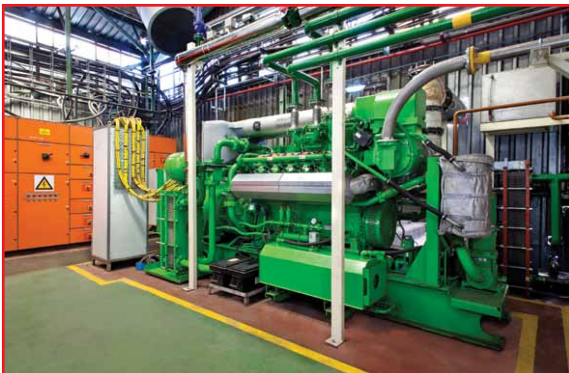
A Jenbacher JMS312 GS-BL engine powered by biogas derived from the anaerobic digestion of fruit waste. Courtesy of Clark Energy
